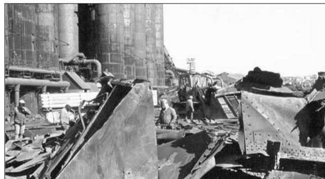
The remains of a steel plant near Pittsburgh, Pennsylvania. Not content with merely shutting plants, the Synarchy is literally dynamiting them to stop the U.S. from any hope of an economic recovery.
