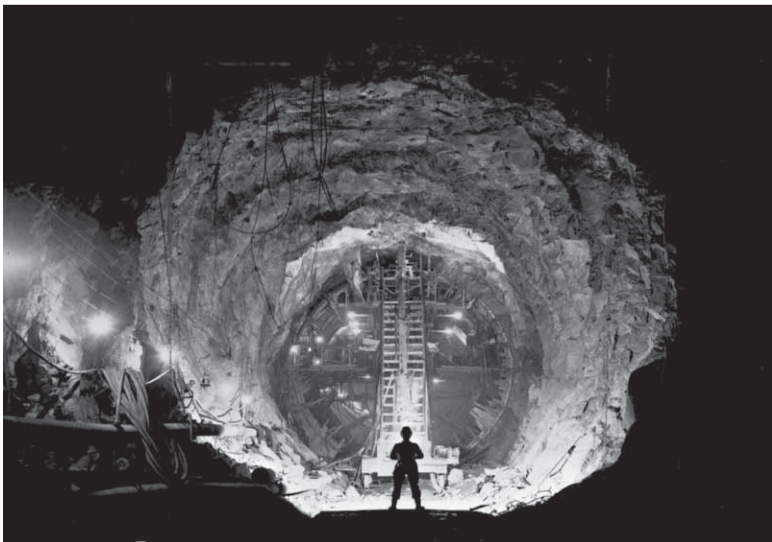
Tunnelling on the Snowy Mountains Scheme, one of the engineering wonders of the world.
